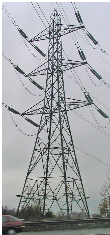
L2 D30 angle tower, Bluebell Hill, Kent
